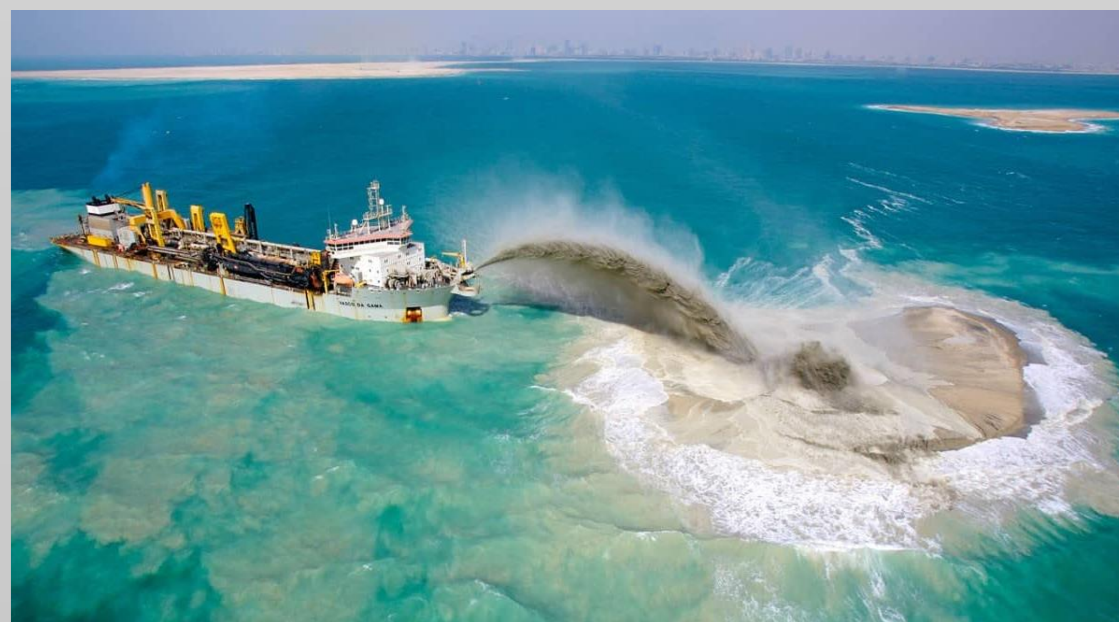
Construction Activities of the Artificial Island using carbonate sand (Dredged from seabed)
